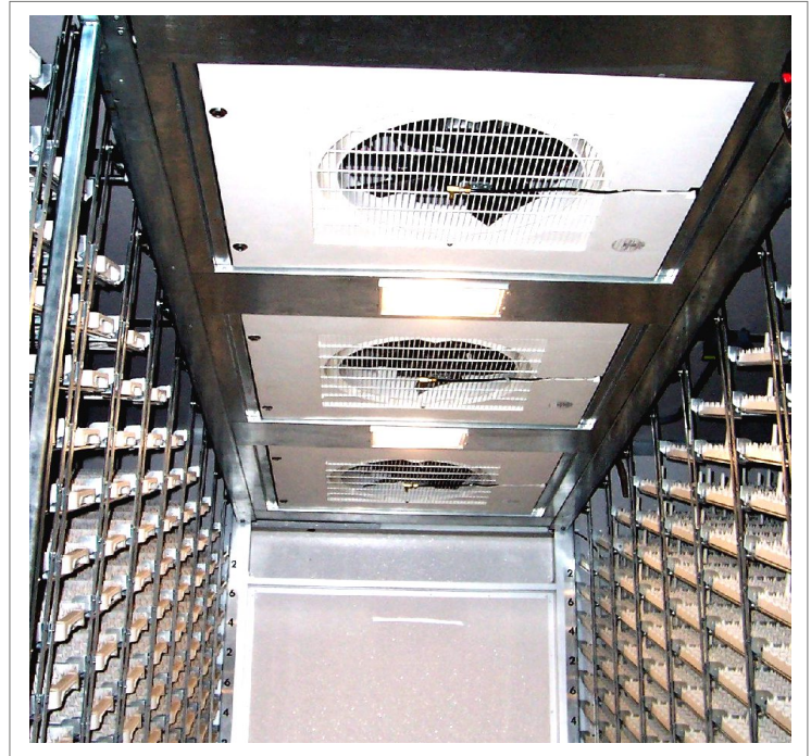
High intensity lighting system mounted between the fan boards
