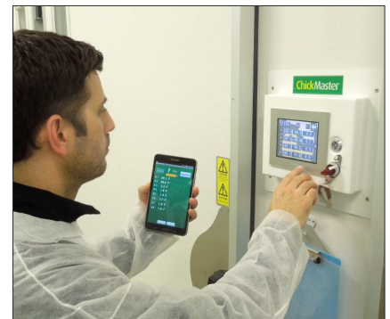
An Android device receives the actual temperature values and allows the technician to make adjustments at the control screen
