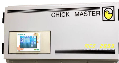
GeMeric 3 installed in existing control cabinet
