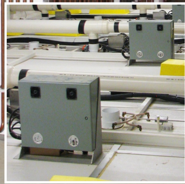
Main picture: Inside the Avida A18 setter showing all three sections Inset: The setter roof mounted Vertical Fan Drive unit
