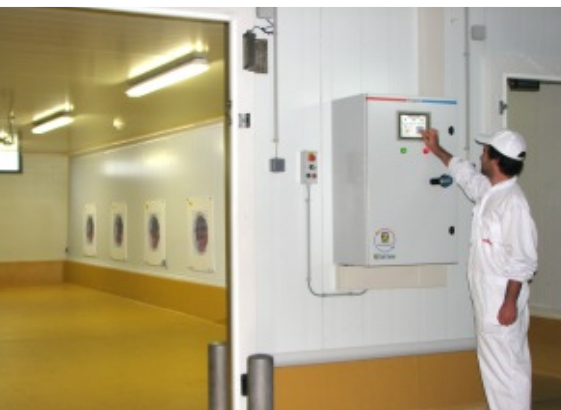
The Lusiaves state of the art 'Lamina Flow' fumigation room
